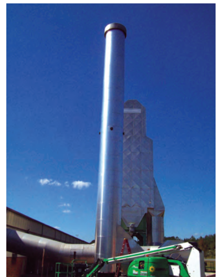
New insulation & lagging installed on customer's exhaust stack, as well as baghouse upgrades during planned shutdown.
