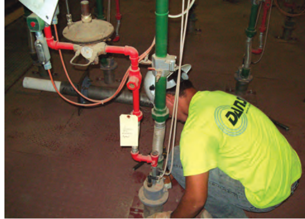
Changing gas burner while the kiln is still running, avoiding expensive downtime for the customer.
